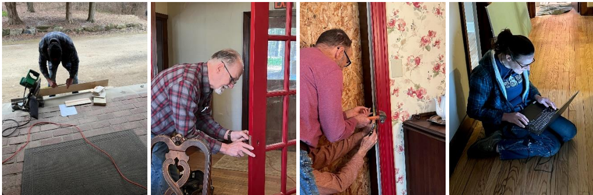
General: Trim being cut for installation. Doug working on the dining room French door hardware. Larry (and Bill) working on the weatherstripping at the exterior door. Corey working on the drawings (mid-measuring). Thank you, Nancy Kanik, for the construction photos!
