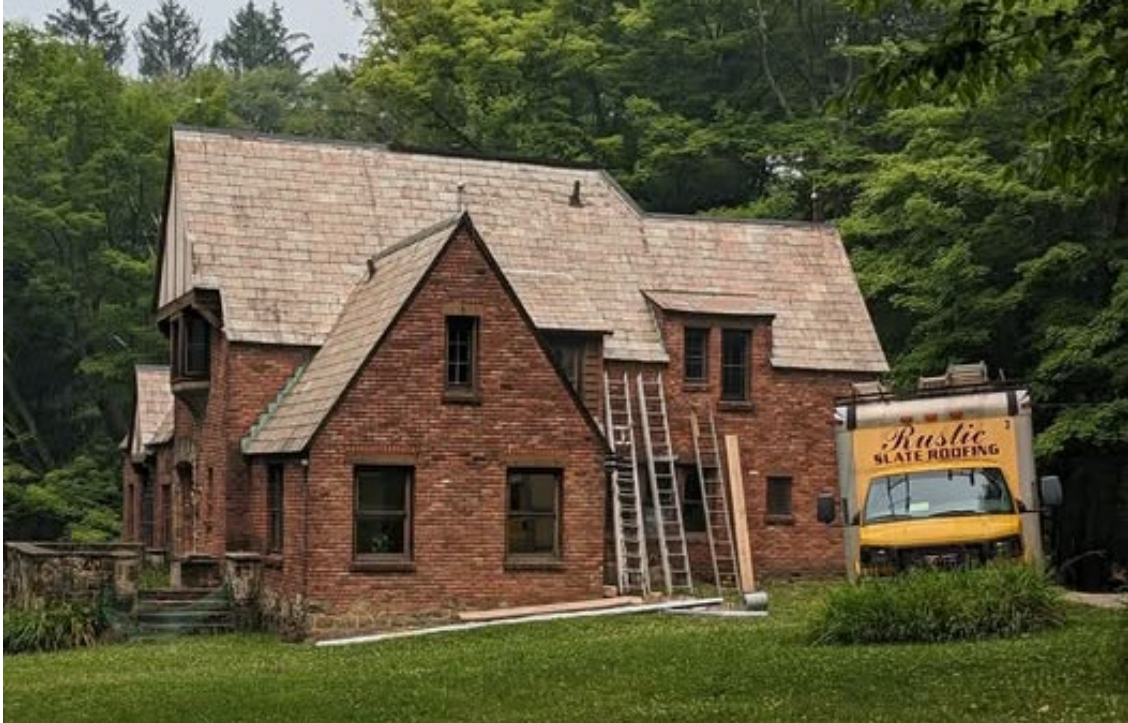
The Friends funded slate repairs, installation of gutters and downspouts at North House
