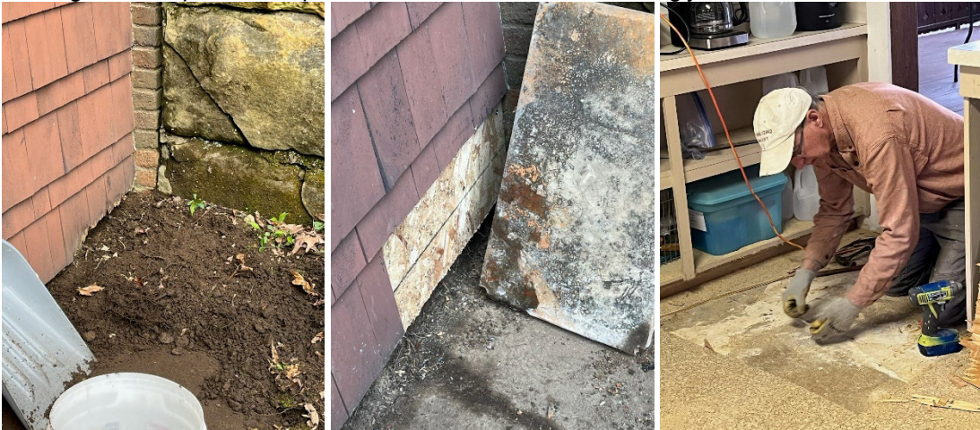
Kirby House Stabilization: Removed damaged gypsum board and batt insulation where animals had started to dig into the garage foundation. Sealed with new sheathing and foam insulation. Removed dirt to prevent moisture from sitting against wood cladding. Started to remove non-original roll out laminate in kitchen. Sub floor in good condition, but finish floor was patched with gypcrete at some point.
