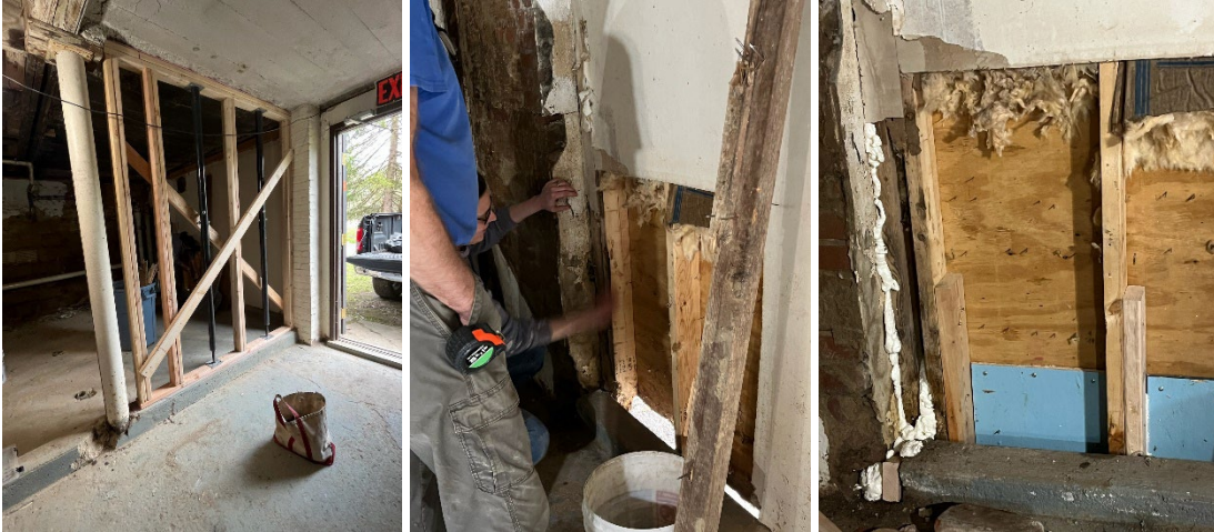
Kirby House Stabilization: Removed showers to investigate concrete slab at kitchen entrance. Concrete haunch removed at some point and concrete starting to fissure and spald. Structural engineer investigated and provided report and recommendations. Bearing jacks / wall installed.
