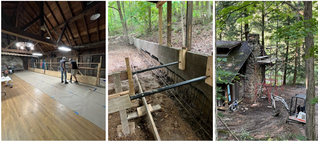
Excavate and trench for the footer, create the formwork, and set reinforcement. Masons working on rear chimney installing new stones, cement wash, and tuckpointing.
