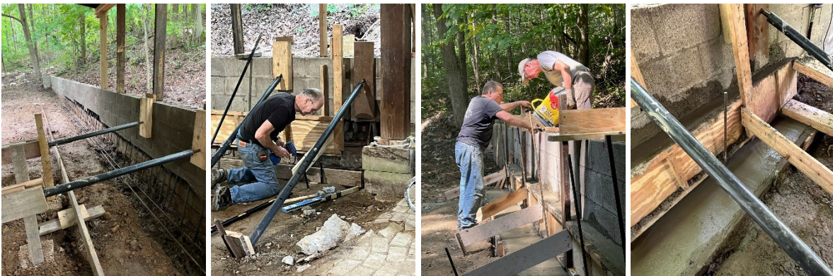
Shoring the CMU retaining wall and adding the rebar, filled cells, and concrete footer.
