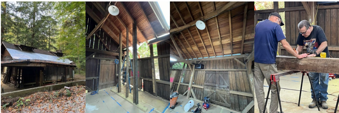
Shoring the timber framing to remove damaged roof sheathing and repair the water damaged top plate timber.
